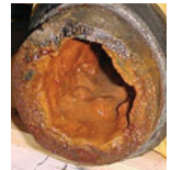
▲ Figure 16.5 A biofilm fouling the insides of a pipe pipes were capable of withstanding levels of chlorine 10 to 20 times higher than the concentrations routinely used to chlorinate drinking water.
